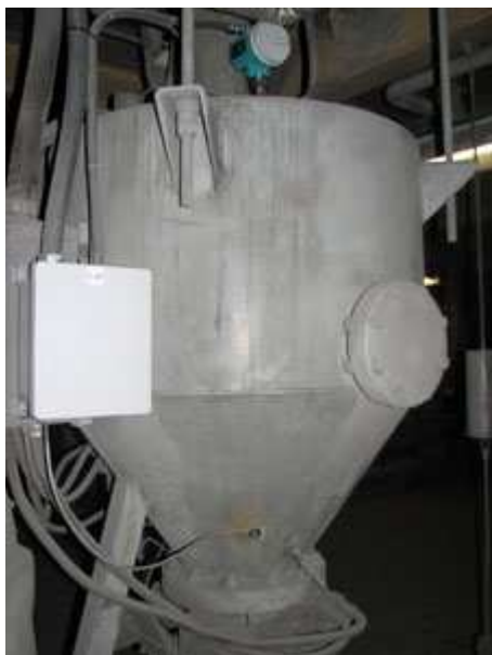
Pressurized feeder with level Transmitter & thermocouple
