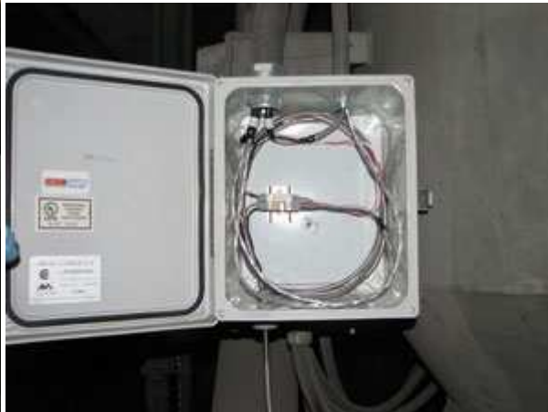
Field wiring box to PLC
